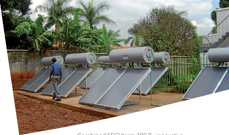
Combined SECUterm 300 P - innovative installation at large Brewery in Uganda
