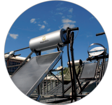
SECUterm at testing facility at the Test Center Saabrücken
